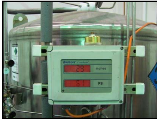
Figure 4 - LN2 Micro-bulk Tank with Barton Cryoscan LN2 tank level digital meter
